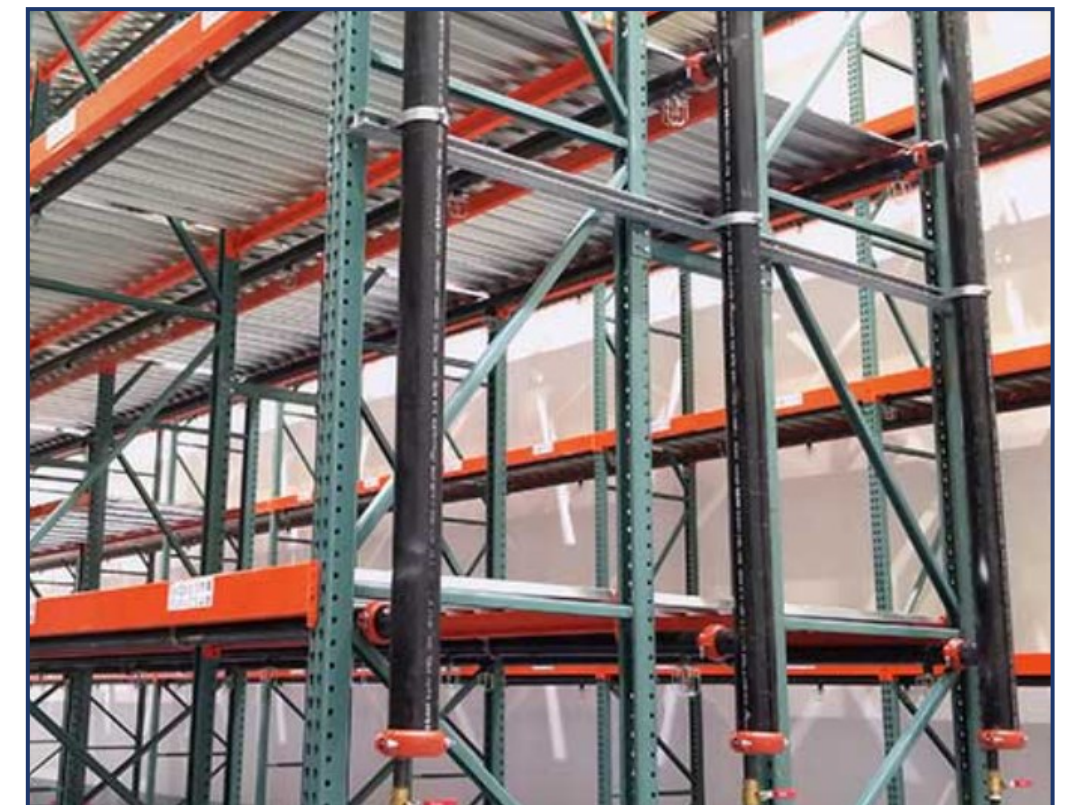
Horizontal steel barriers separating levels of storage Shown with installed double-row rack sprinklers
