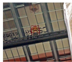
ESFR-rated in-rack sprinklers with steel barriers between storage levels
