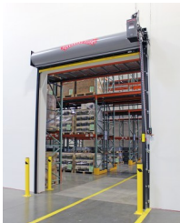
2-hour fire-rated containment walls and steel door
